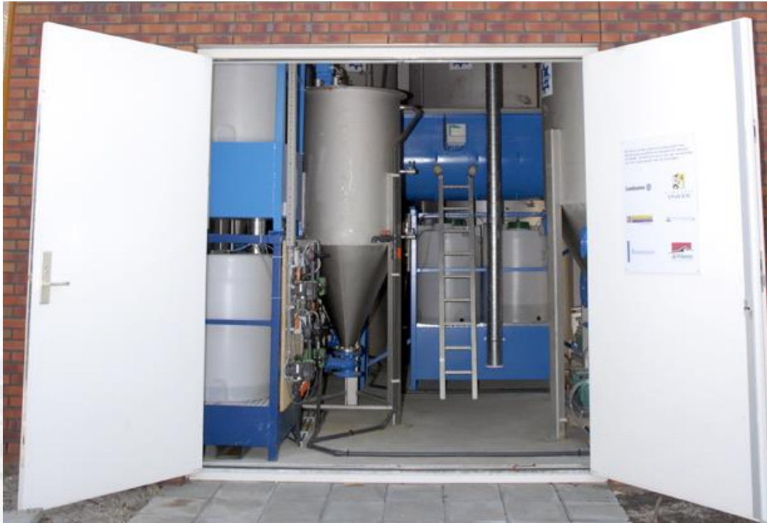
2005, 32 houses with vacuum toilets
